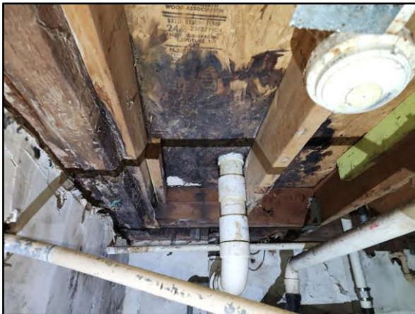
Visible mold on OSB ceiling board and framing in basement storage room 2.
