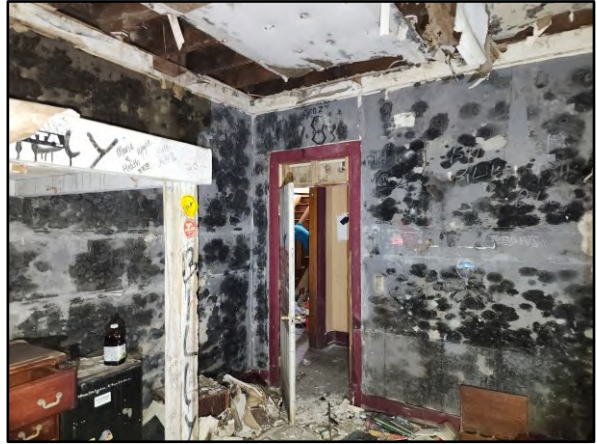
Visible mold on the walls and ceiling of Bedroom 4 on the first floor.
