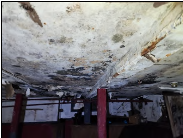
Mold on the drywall ceiling in the basement.
