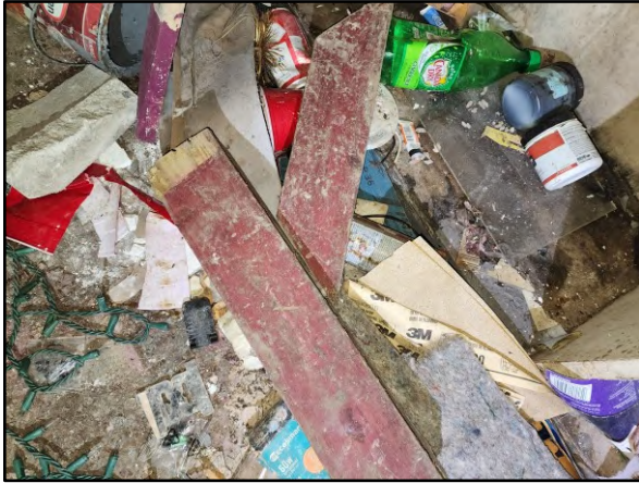
Debris on basement floor with visible mold.
