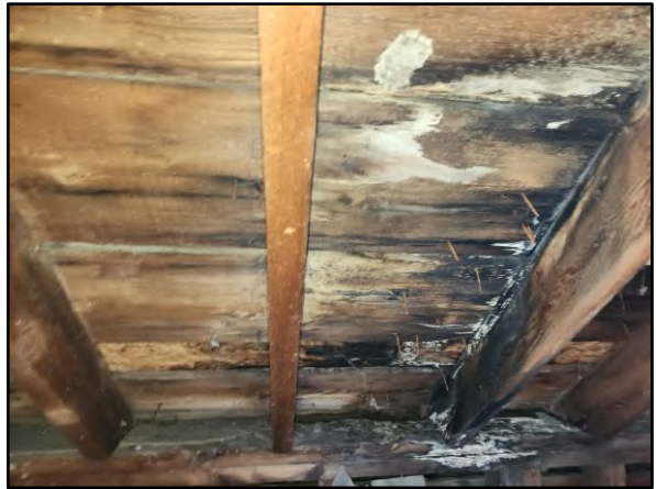
Visible mold on the roof decking and framing in the attic.
