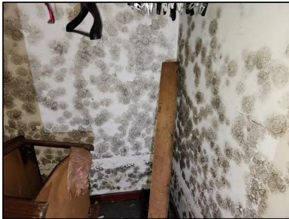
Visible mold in the closet of Bedroom 9 on the second floor.
