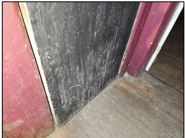
Visible mold on wood door on the first floor.
