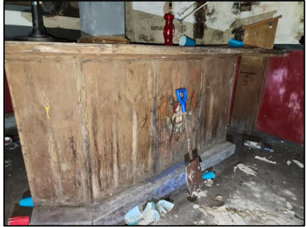
Bar in basement dining room with visible mold.
