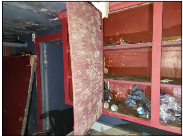
Basement cabinets with visible mold.
