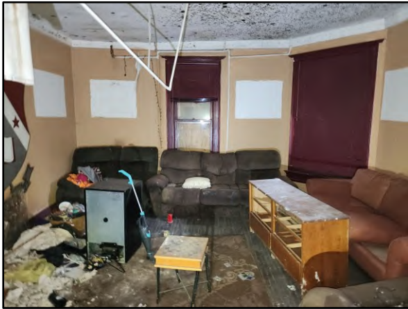
Visible mold on the ceiling of the first floor living room.
