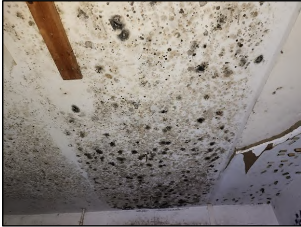
Visible mold on the ceiling of Bedroom 3 on the first floor.
