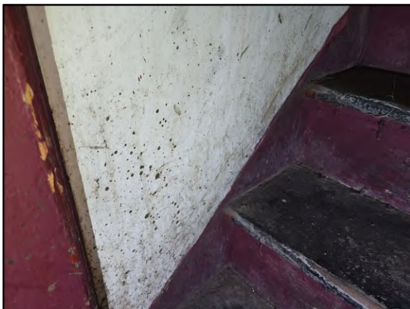
Visible mold on drywall wallboard at back stairs.
