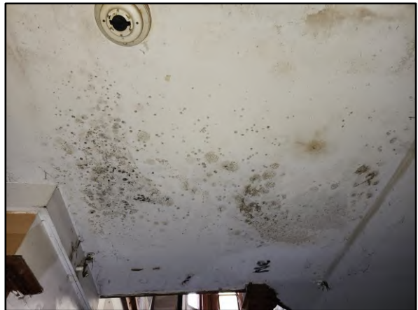
Visible mold on the ceiling of the first-floor entry foyer.
